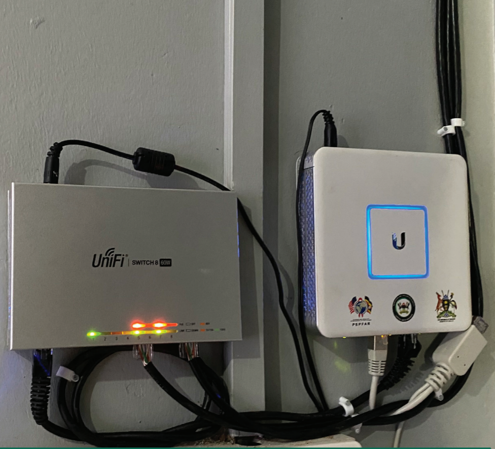
Point Of Care (POC) Equipment installed in Koome Health Center IV
