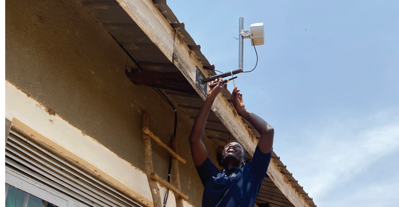
TSS ICT Service Analyst installs antenna to boost network connectivity at Kawongo HC II
