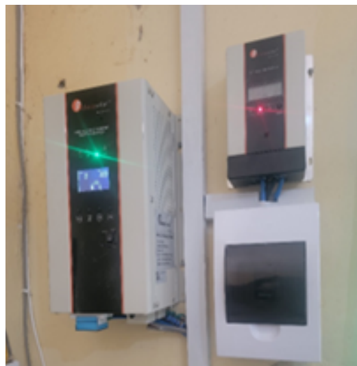
Solar Control Panel Installed at Busabaga HCIII in Buikwe
