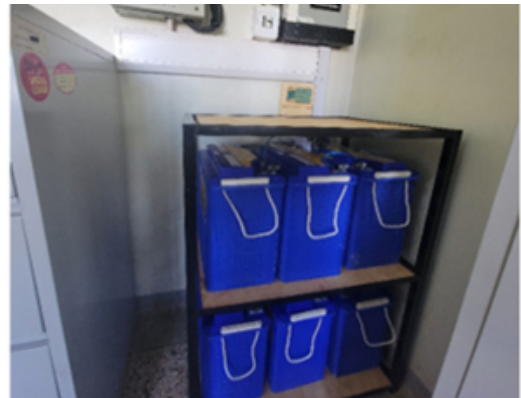
Solar Batteries Installed at Lugasa HCIII in Kayunga
